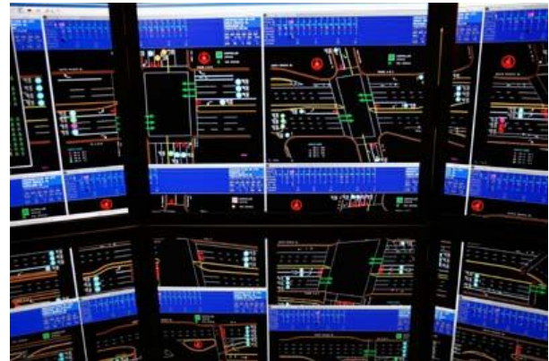
Figure 2 Machine-to-machine communications can be used to monitor traffic in real time, like at this Los Angeles traffic center.
